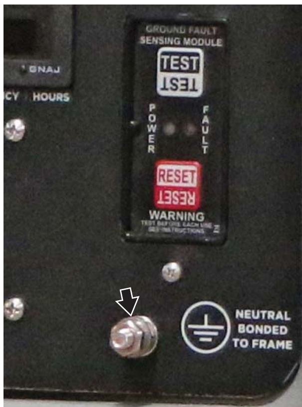
Figure 16 – Ground Terminal on the Control Panel
