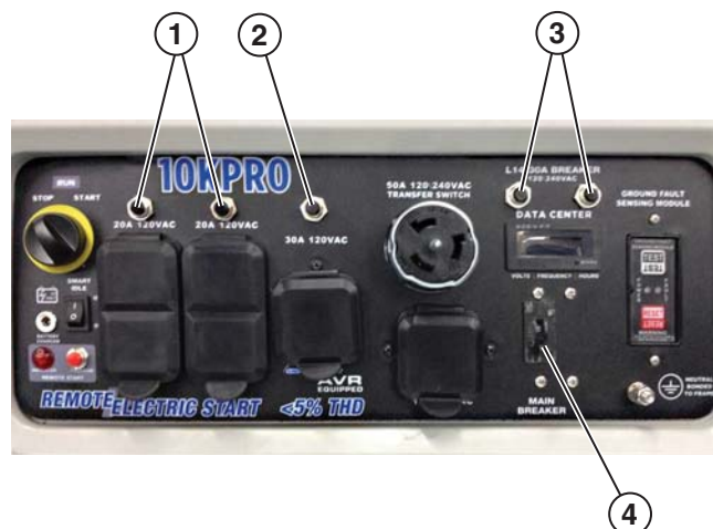
Figure 25 – Circuit Breakers – 10KPRO
