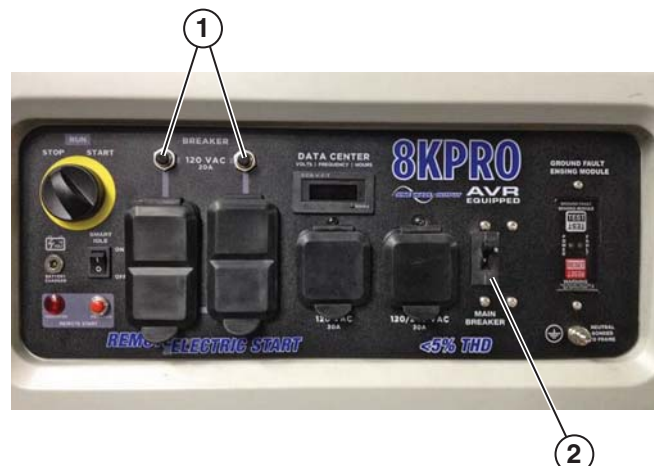
Figure 26 – Circuit Breakers – 8KPRO
