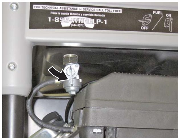
Figure 31 – Fuel Shutoff Valve in the ON Position
